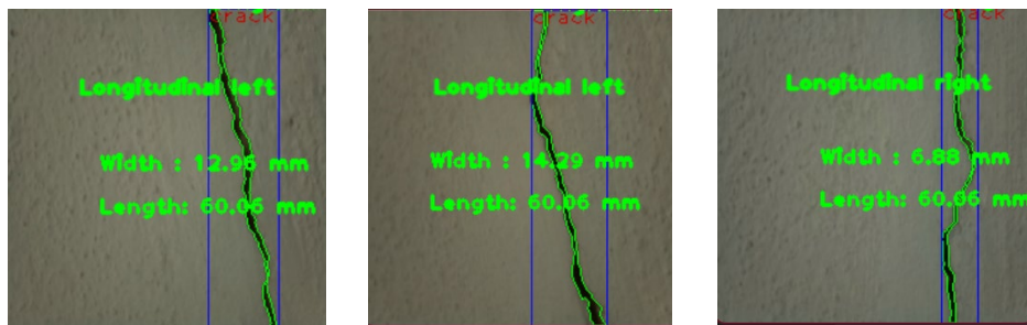
Figure 14. Longitudinal crack detection results.
