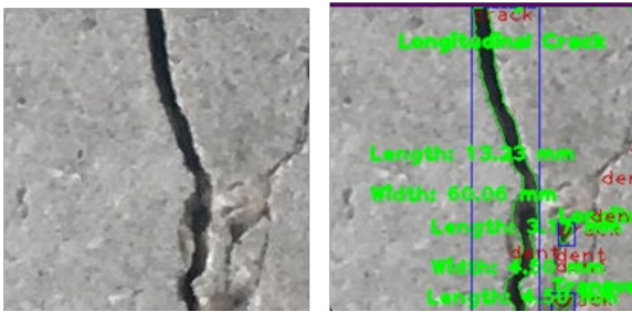
Figure 18. Tiny crack fails to detect.
